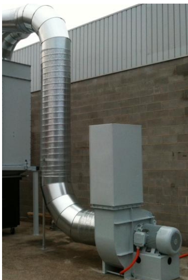
Multiple motors or Ground mount fan
